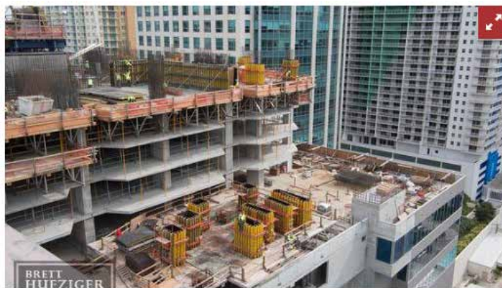
The first four floors of the apartments at Panorama Tower have been poured atop the parking garage.
